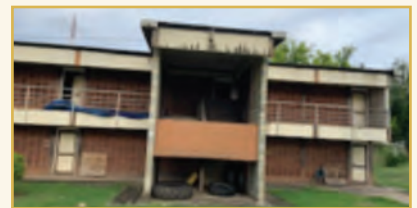
An overview of the condemned building
